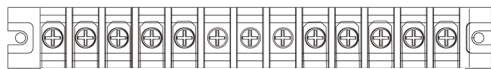
Fig. 35. Detail of connection terminals configuration Input-Output configuration: three-phase-three-phase with common bypass line.
