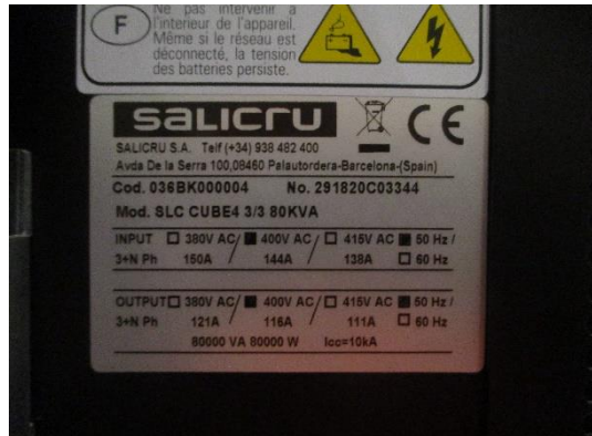
Factory Identifier label (tested equipment)
